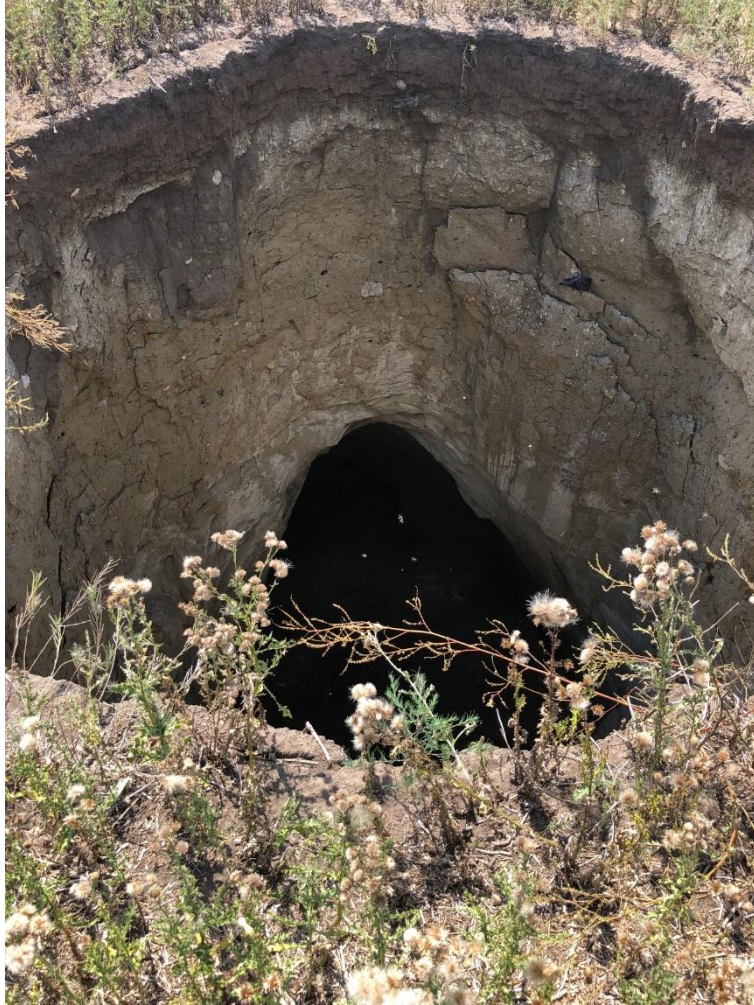
Figure 1: This large dangerous sinkhole opened up near a trail on the edge of a cropland field.
