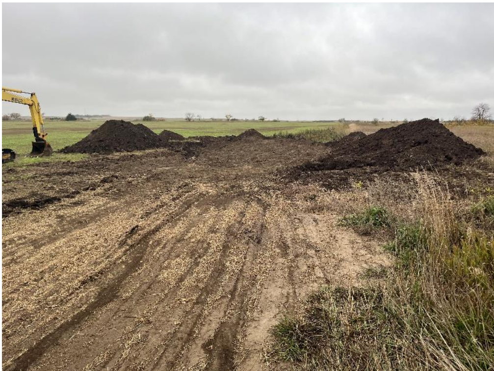
Figure 2: The sinkhole was filled and is about to be respread with topsoil.
